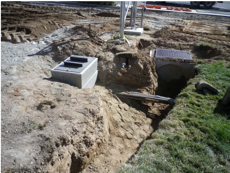
New gate controller junction box installed
