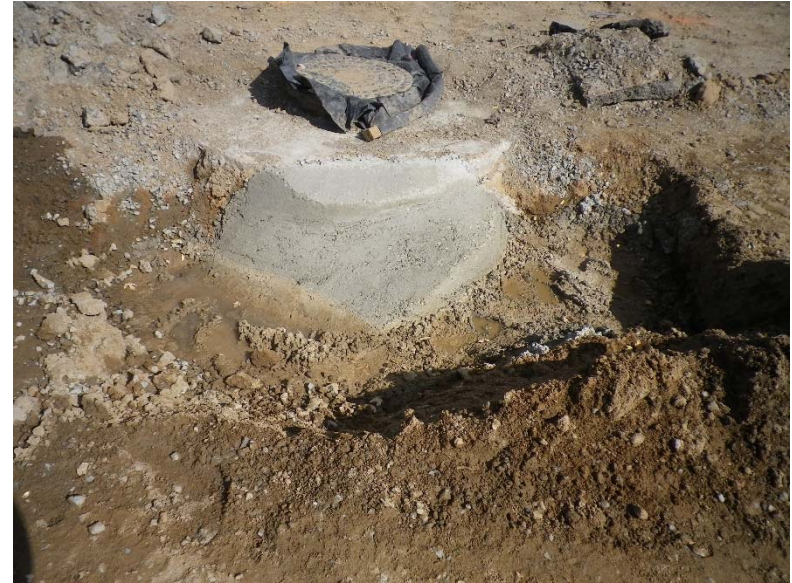
Unforeseen circumstance – previously damaged manhole cover
